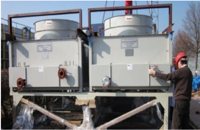
Dummy Load Heat Exchange installed by M/s Thomson Engineers at France
